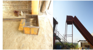
Fig 1 :- A View of Inlet Tank
